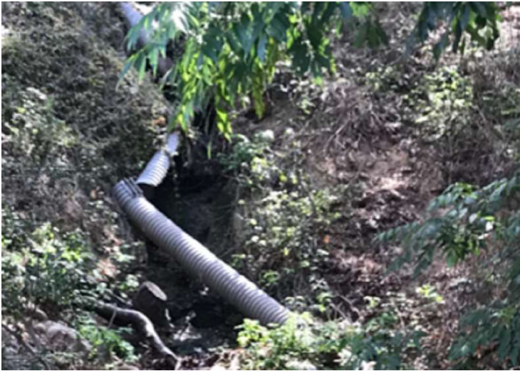
Damaged Storm Drain
